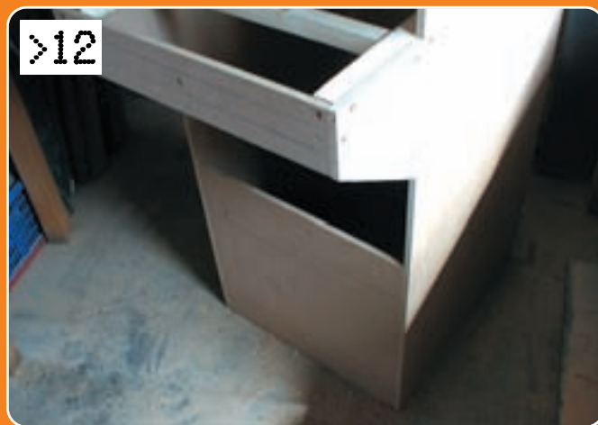
>12 It's worth adding an additional internal brace. Then it's time for a front panel, constructed in much the same way as the back panel. This doesn't come all the way up the front of the case, because we're going to add a door above it so that we can access the internal PC components when necessary.
