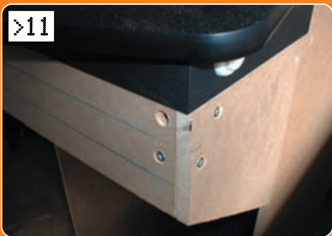
>11 A cross-brace can now be added underneath the controller. Again, this has batons attached to it and we'll screw through the sides into these batons, holding the cabinet together and supporting the controller securely into the bargain. Although we've not done it yet, it's a good idea to drill into the cross-brace in two places, so it won't move around.
